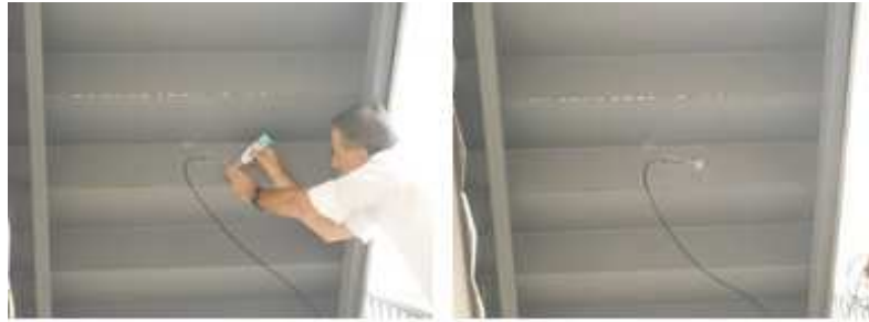
FIGURE 4. Accelerometer installation on the bottom side of the stairway.
