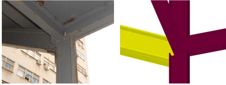
FIGURE 11. Eccentricity of beam elements at a common node: (left) actual connection; (right) FEM model representation.
