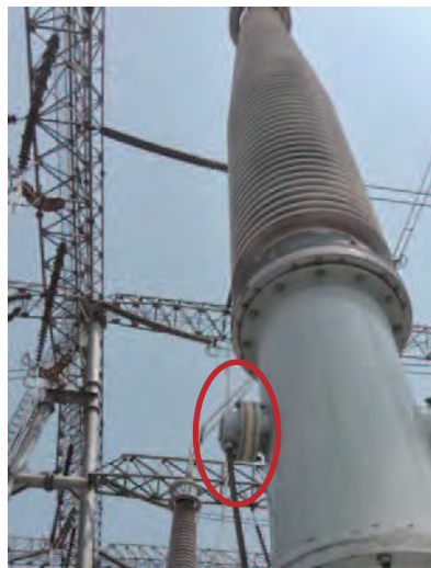
Figure 11: Insulation of the live display device of the 5062C-2 Knife Gate gas chamber
